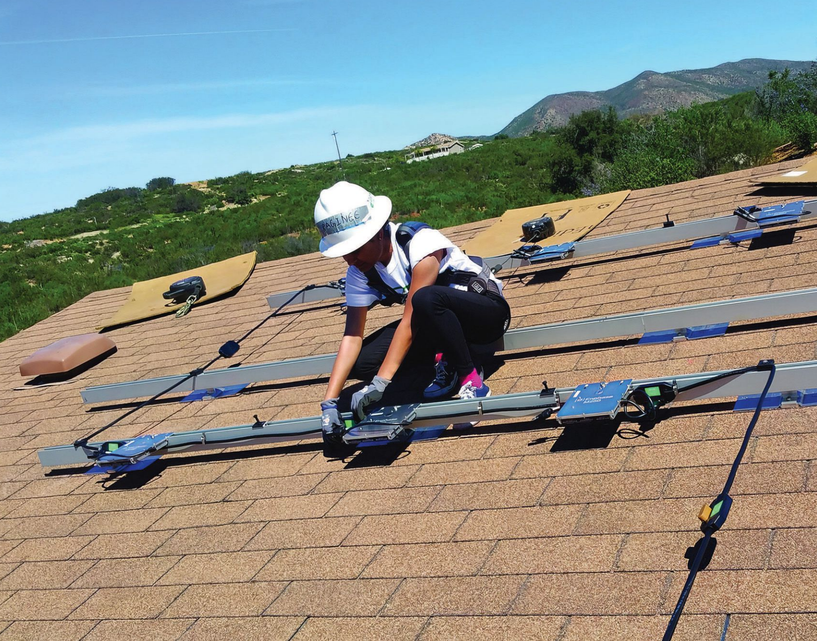
Solar installers work long hours on rooftops preparing supporting hardware and other components of renewable energy systems.
